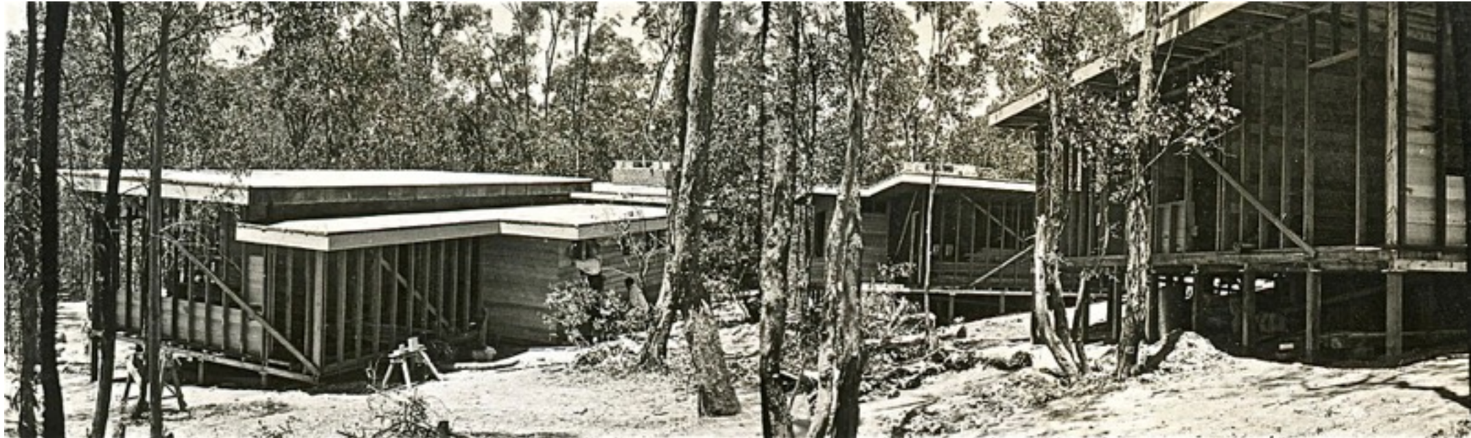
Construction begins. Flat asbestos cement roofs. The class rooms were framed up with timber studs left exposed. These were later painted cream.
